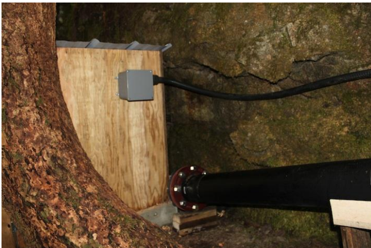
Figure 7 - Turbine house built on rock ledge and protected from washout by a tree.
