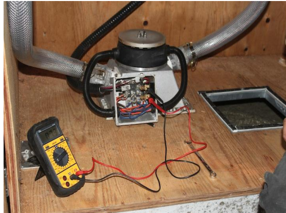
Figure 6 - Turbine installed in turbine house. Water enters through the two clear pipes and drains out under the turbine.
