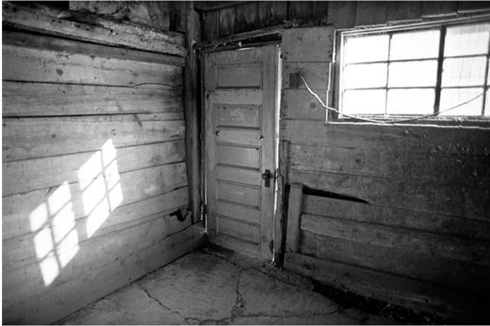
An interior view of a storage room in the barn, seen after the author finished clearing a stack of old bricks from beneath the window.
